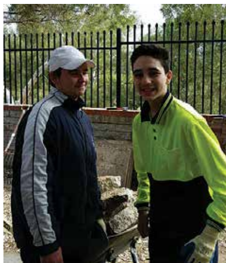
Year 9 students, Marko Simovic and Keanu Rhoades working onsite preparing their worksite to build herb gardens
